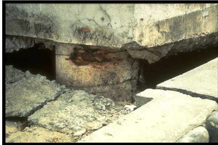
Fig. 4.8.3 Example of damage at the pile-cap connection
